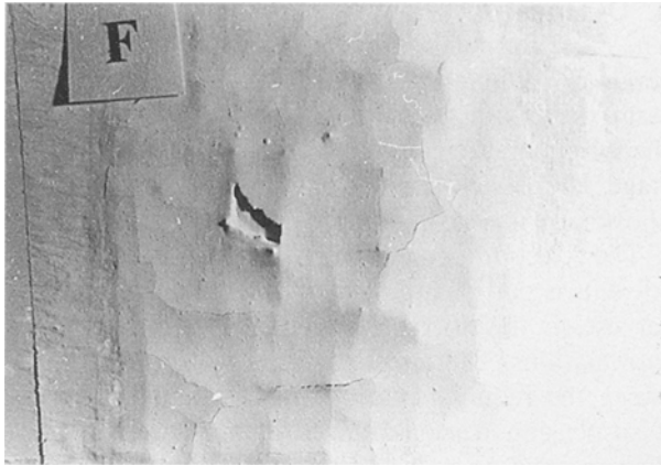
Figure 2 Paint films of composition 2 deposited by brushing showing the cracks that appeared on drying.
